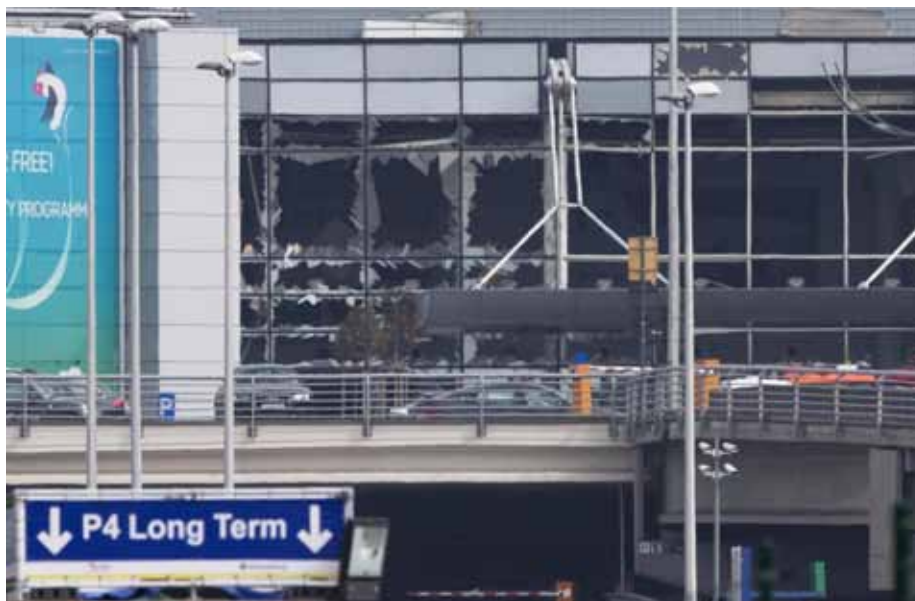
The blown out windows of Zaventem airport are seen after a deadly attack in Brussels, Belgium, on Tuesday, March 22, 2016.
