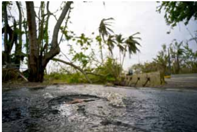
This Thursday, October 12, 2017 photo shows an overflowing storm drain, in Dorado, Puerto Rico.
