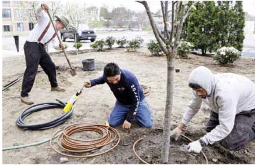
In this April 25, 2017 photo, Stephen Faulkner, far left, owner of Faulkner's Landscaping & Nursery, installs an irrigation system alongside workers Gonsalo Garcia, center, and Jalen Murchison, right, at a landscape project in Manchester, New Hampshire.
